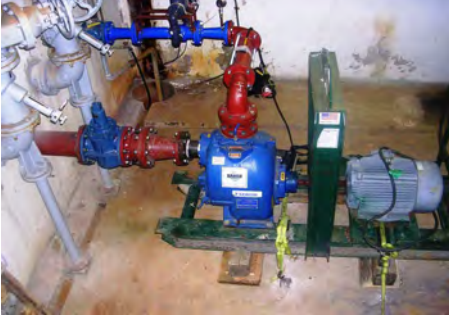
Eliminating H 2 S in a lift station & Main
