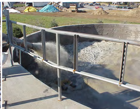
Aeration Septage—Eliminating H 2 S & reducing BOD
